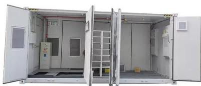
1075KW HH ESS
