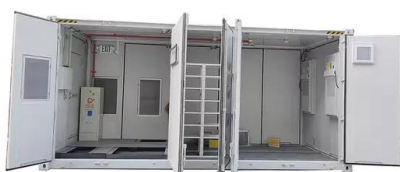
1075KW HH ESS
