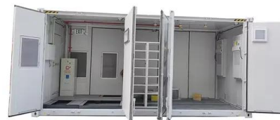
1075KW HH ESS
