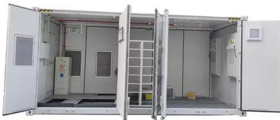
1075KW HH ESS
