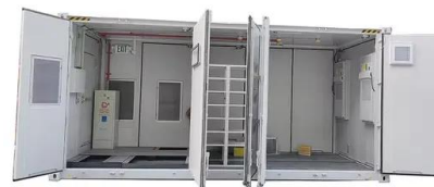
1075KW HH ESS
