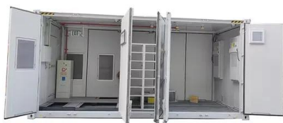
1075KW HH ESS
