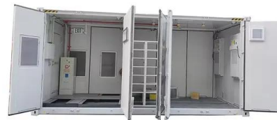
1075KW HH ESS
